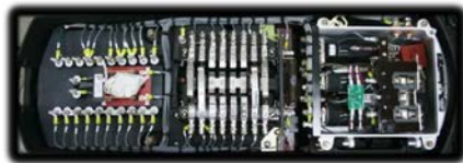
Alstom 5H Contact Compartment
